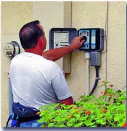
Controller with wrong watering schedule?
