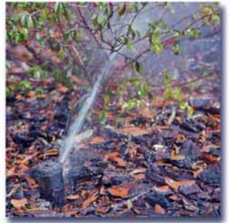
Wrong spray heads?
